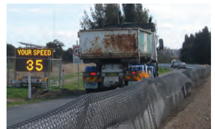
Pictured: A variable message board is in place in the construction area to show drivers their speed.
