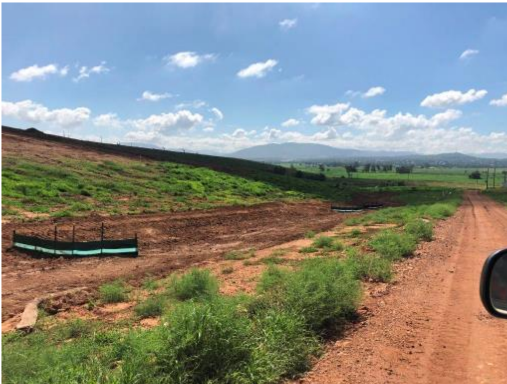
Erosion Photo 2 - Sediment fences within the drain may fail as sediment fences have been used in an area of concentrated flow
