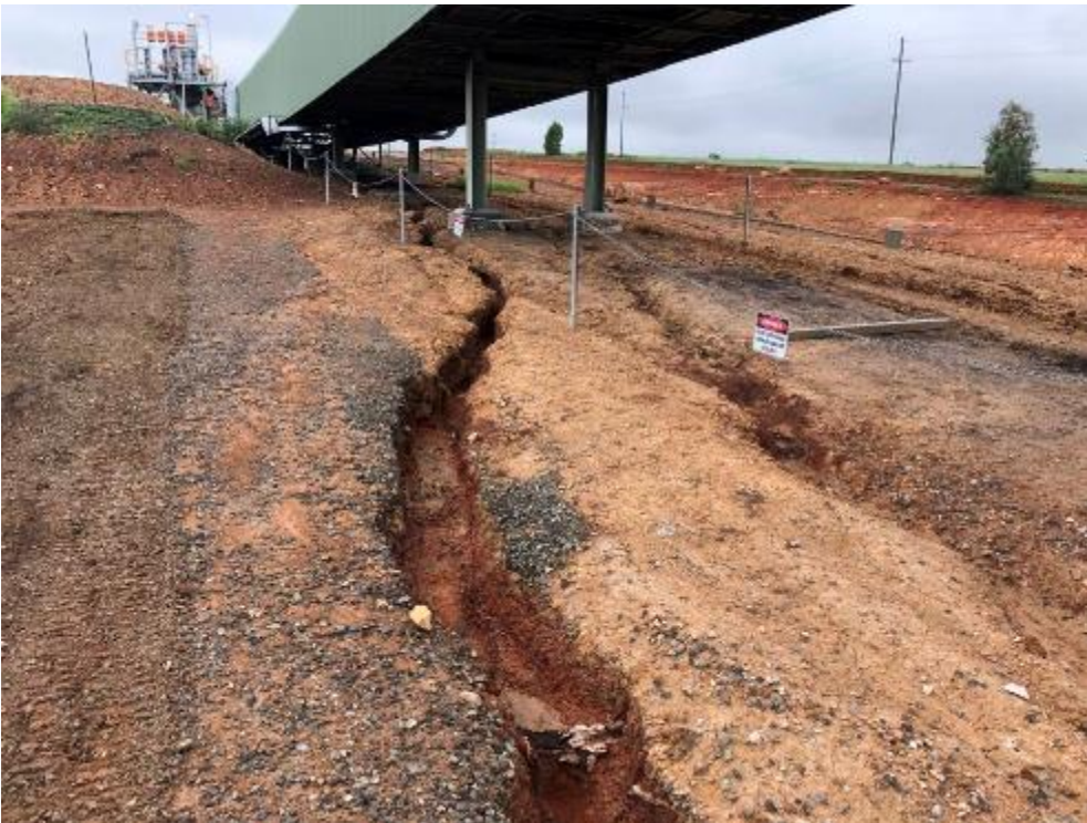
Erosion Photo 4 - Erosion along the roadway to the Train Load Out Area. Note – Evidence provided that erosion issue has been remediated, however maintenance is ongoing
