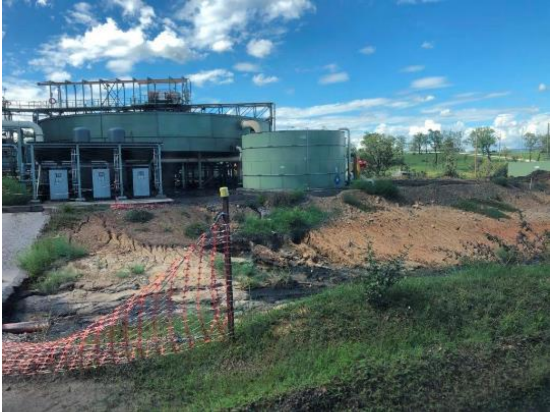
Erosion Photo 7 - Erosion in the CHPP Area. Some works have completed since the site inspection (April 2020) but ongoing maintenance is required.
