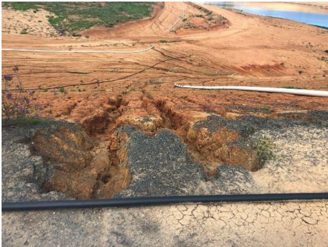
Erosion Photo 12 - Erosion of the inside of the wall of the fines emplacement area
