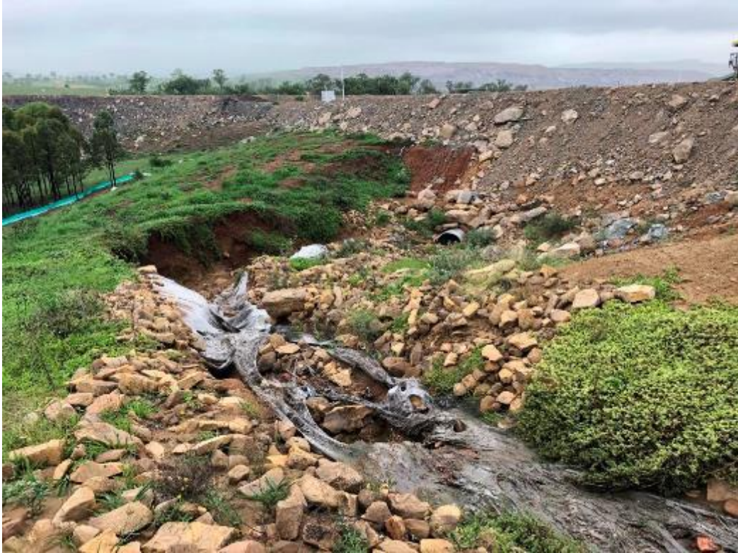
Erosion Photo 3 - Rock lined drain near the pit top has failed and needs full redesign and rework
