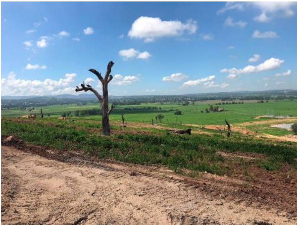
Rehabilitation Photo 2 - Area recently shaped and seeded. Cover crop is well established
