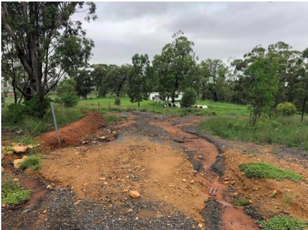
Erosion Photo 14 - Erosion near construction offices
