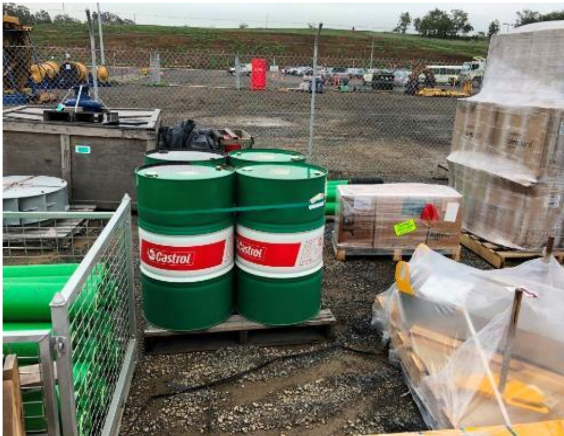
Waste Photo 6- Workshop Area. 44 gallon drums containing oil have not been stored within bunds
