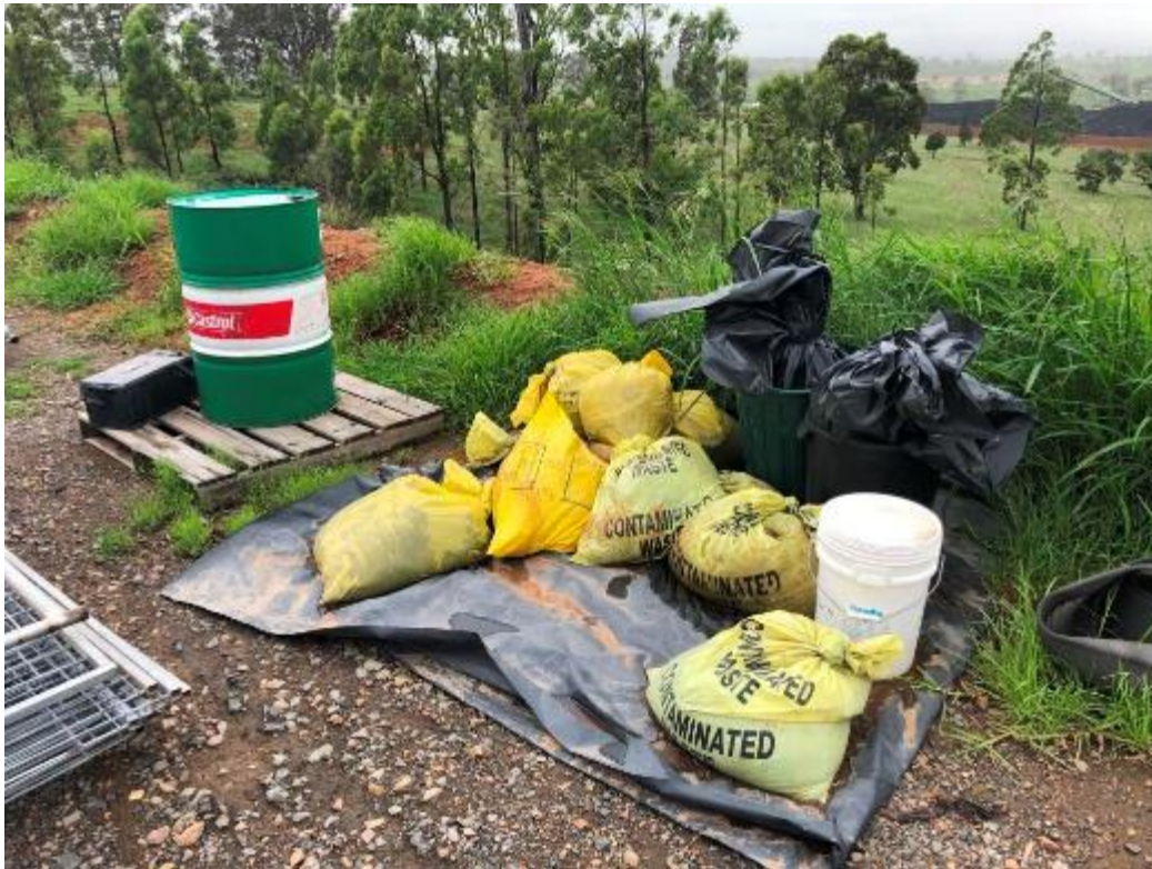
Waste Photo 7 - Construction offices. Drum not stored in bund. Contaminated soil has not been moved to the landfarm. Evidence provided since site inspection that this has been completed.
