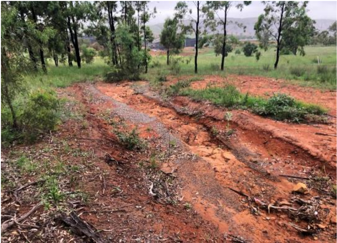
Erosion Photo 13 - Erosion near the construction offices
