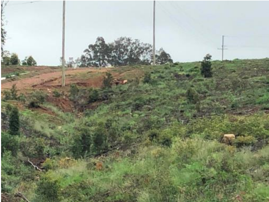
Erosion Photo 5 - Two power poles at site appear to be affected by erosion
