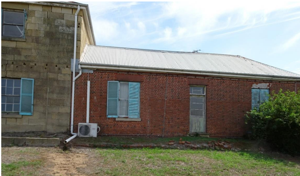
Figure 11. The southern elevation of the c.1845 brick section of Negoa. Note the Flemish bond brickwork of this original c.1845 section. Photograph taken April 2018.
