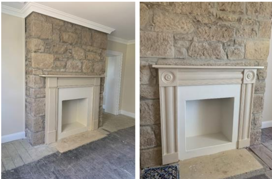
Figure 40. The exposed repointed stone chimney breast and reinstated fireplace and mantelpieces in the upstairs bedrooms.
