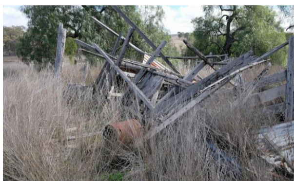
Figure 11. The remains of the cow bails at MP27, constructed of timber and corrugated iron (Source: Extent Heritage 2020, p. 94).
