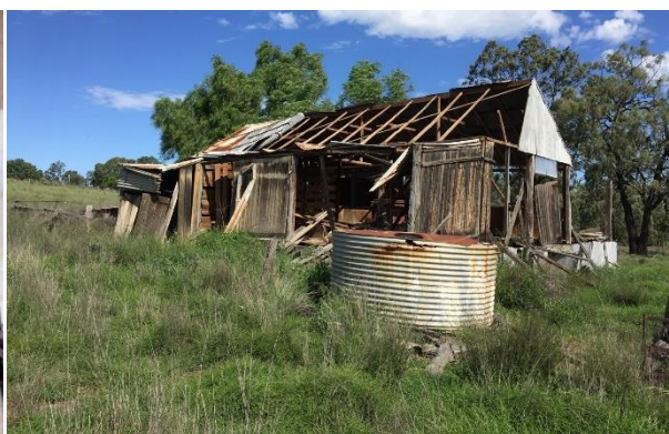
Figure 9. The damaged remains of the shearing shed at Thorndale (MP27) in early 2019 (Source: MACH 2019 in Extent Heritage 2020, p. 93).
