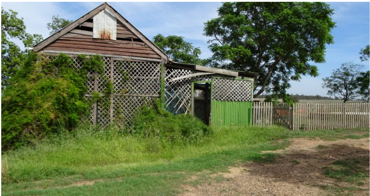
Figure 21. The servants' quarters, showing the extension constructed of timber and corrugated sheet metal. This photograph shows the building as it was in April 2018.
