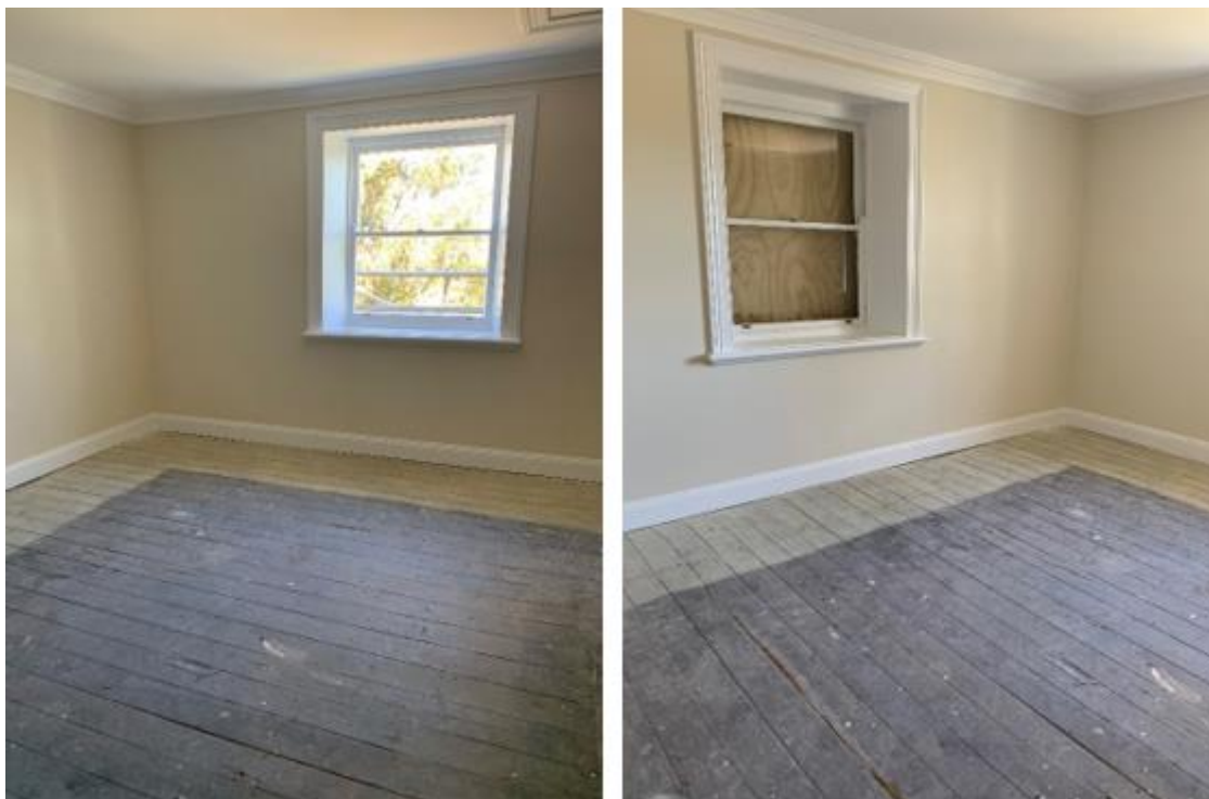
Figure 41. View of the new reconstructed windows, reconstructed to original detail and profile.
