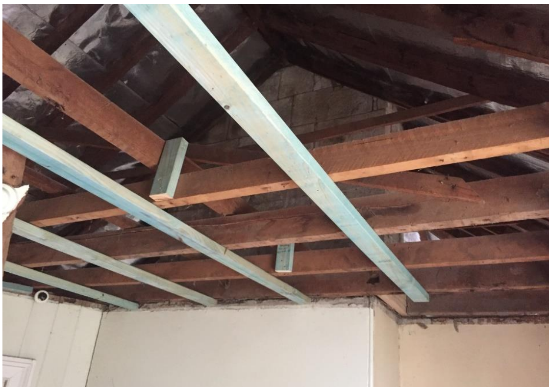
Figure 32. Image illustrating the ceiling space in one of the upstairs rooms showing the augmentation of the roof structure following the removal of the dilapidated ceiling fabric.
