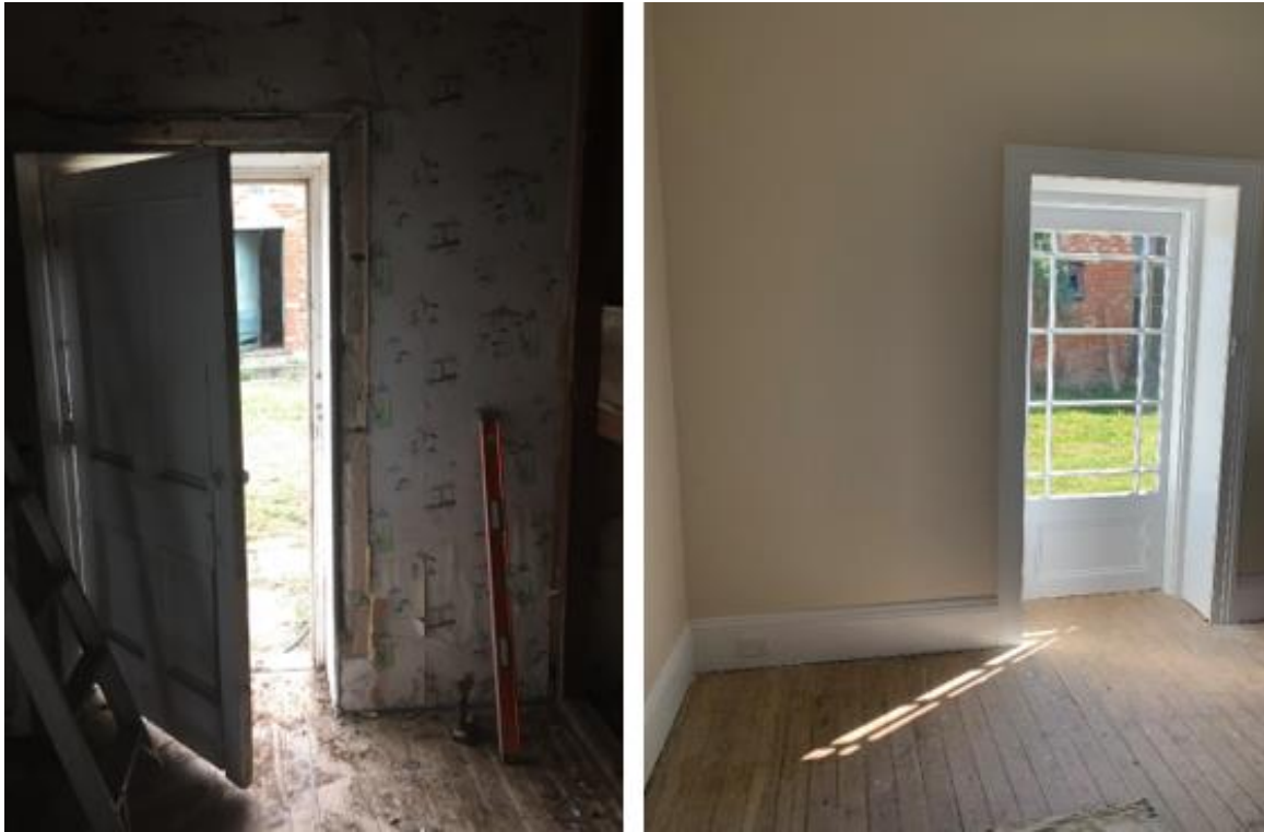
Figure 36. Left: The original four-panel entry door, which has been removed. Right: The replacement half-glazed door with margin glazing.
