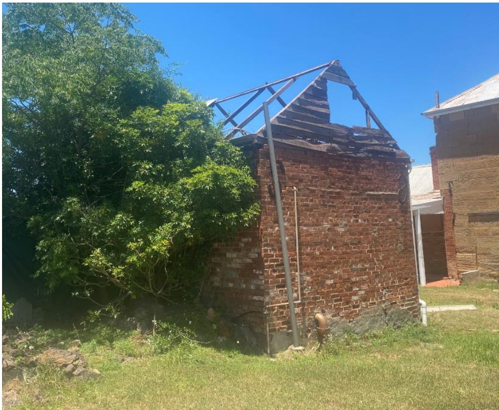
Figure 23. The western elevation of the servants' quarters, showing the damage sustained to the roof as a result of a storm event in December 2020.
