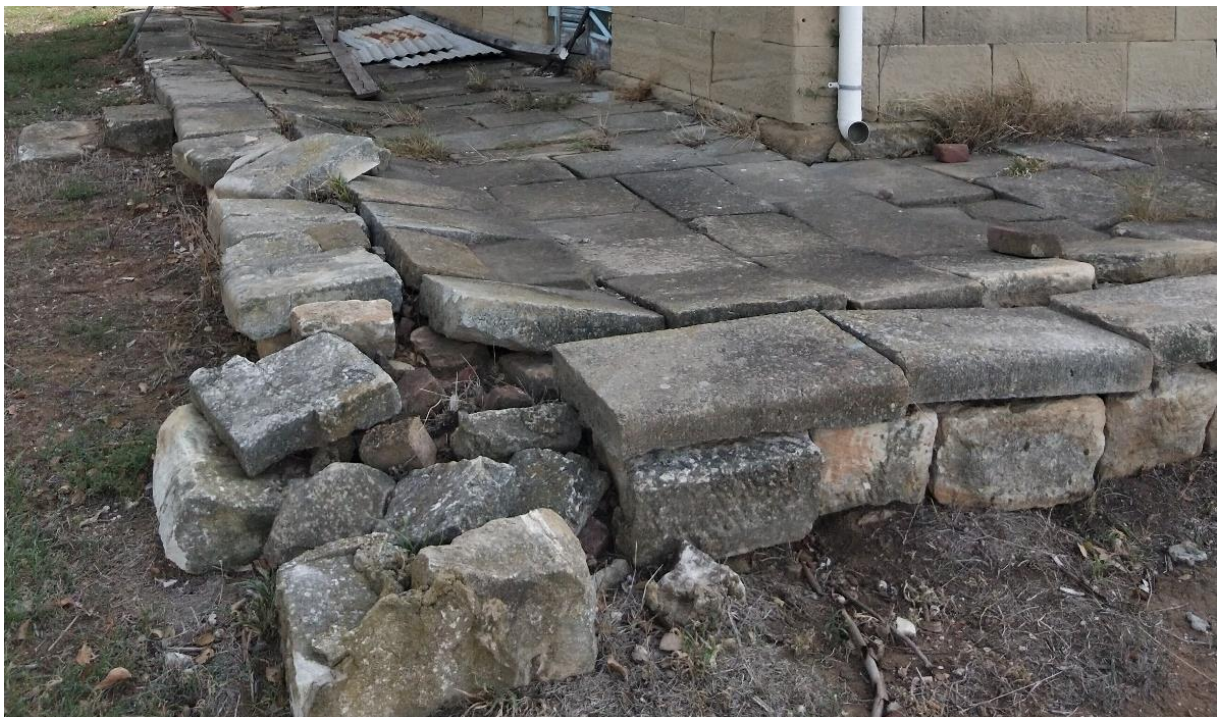
Figure 16. The failed stone paving on west and north elevations of the c.1850s–60s sandstone section of Negoa. Photograph taken April 2018.
