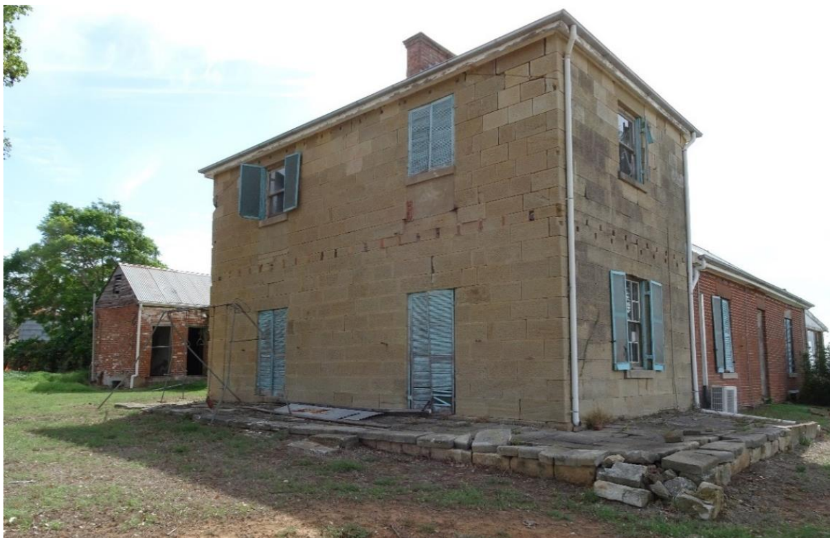
Figure 10. The western elevation of Negoa's sandstone section. Note the holes in the sandstone where the verandah was originally mounted. The servants' quarters are visible to the left and the c.1845 brick section of the homestead is visible to the right along the southern elevation. Photograph taken April 2018.
