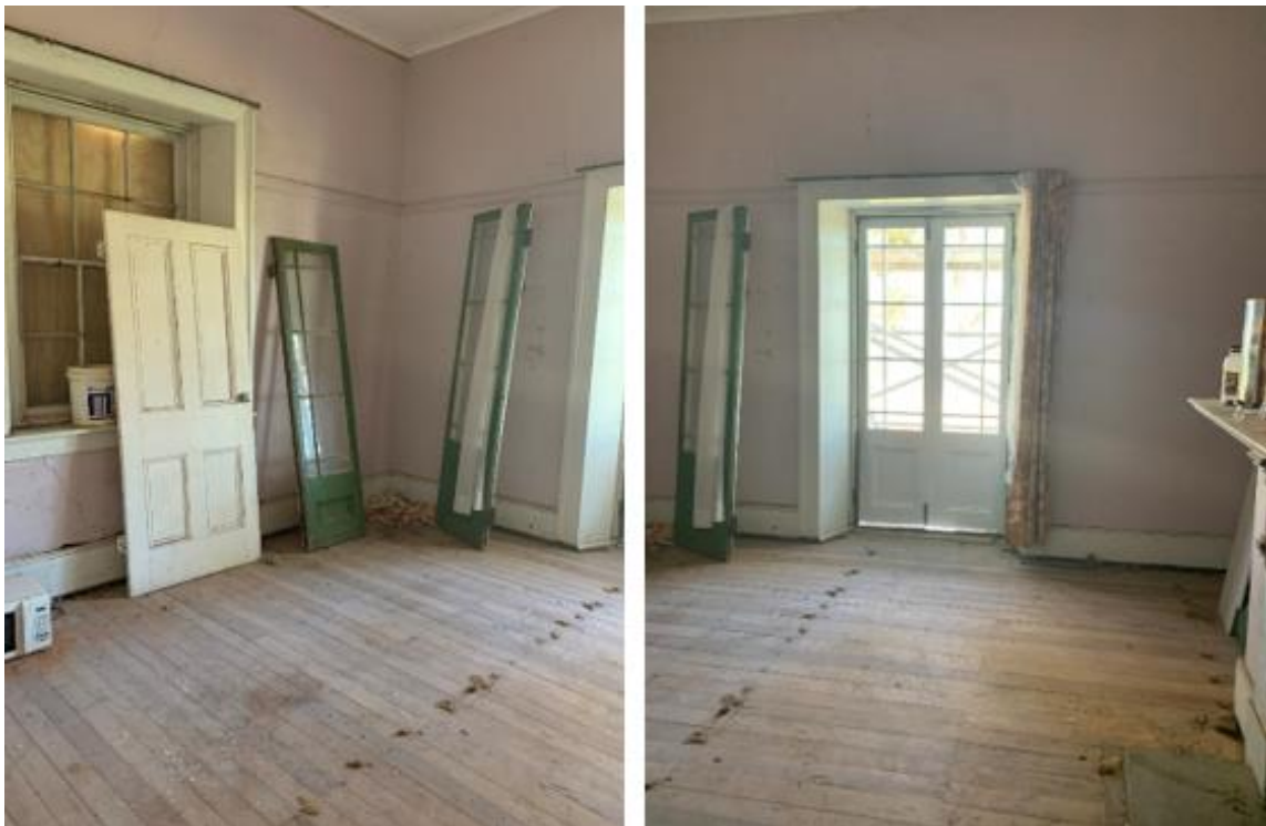
Figure 37. Left: The removal of the existing French doors. Right: The reinstatement of new doors reconstructed to the original profile.
