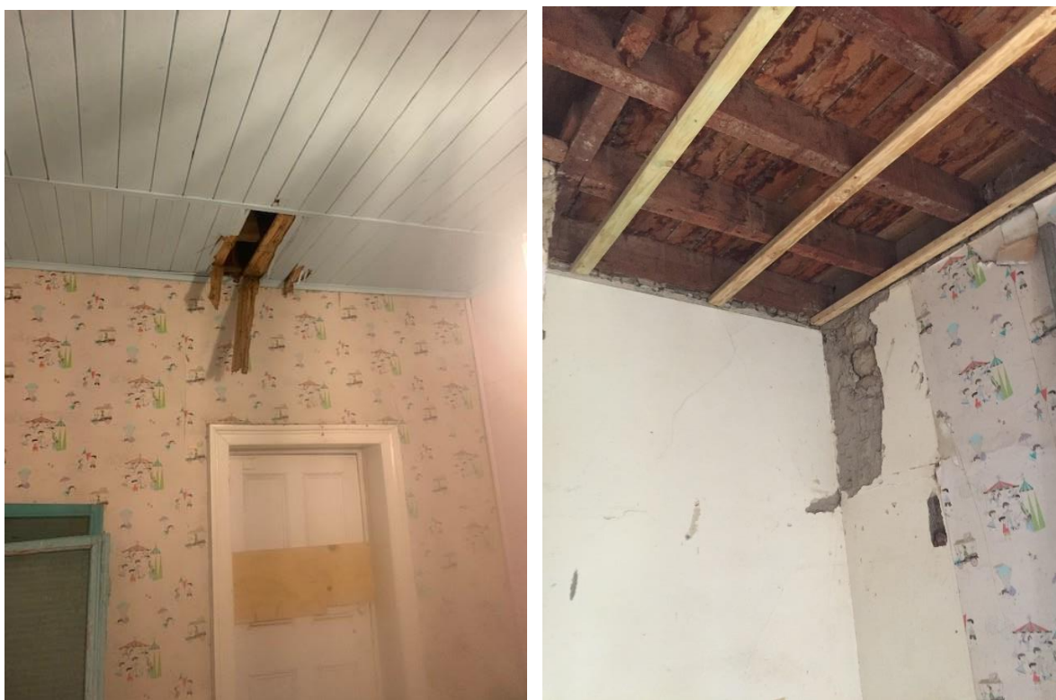
Figure 33. Details of the termite-damaged ceiling removed from the downstairs bedroom.
