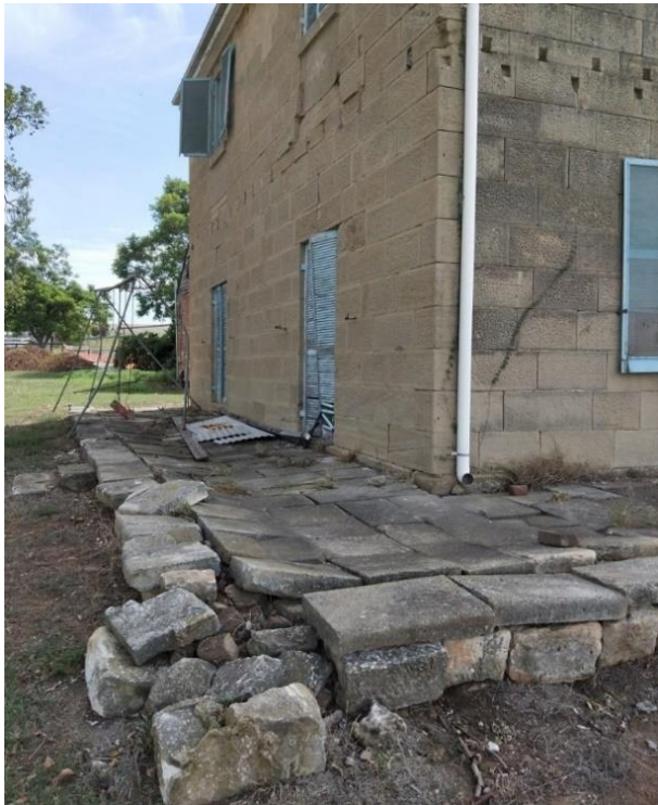
Figure 52. A section of the failing stone paving on western and northern elevations of the sandstone section of Negoa.
