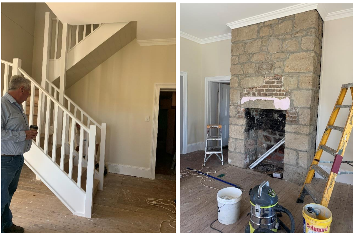
Figure 35. Left: The reconstructed internal stair. Right: The exposed stone chimney breast in ground floor bedroom.
