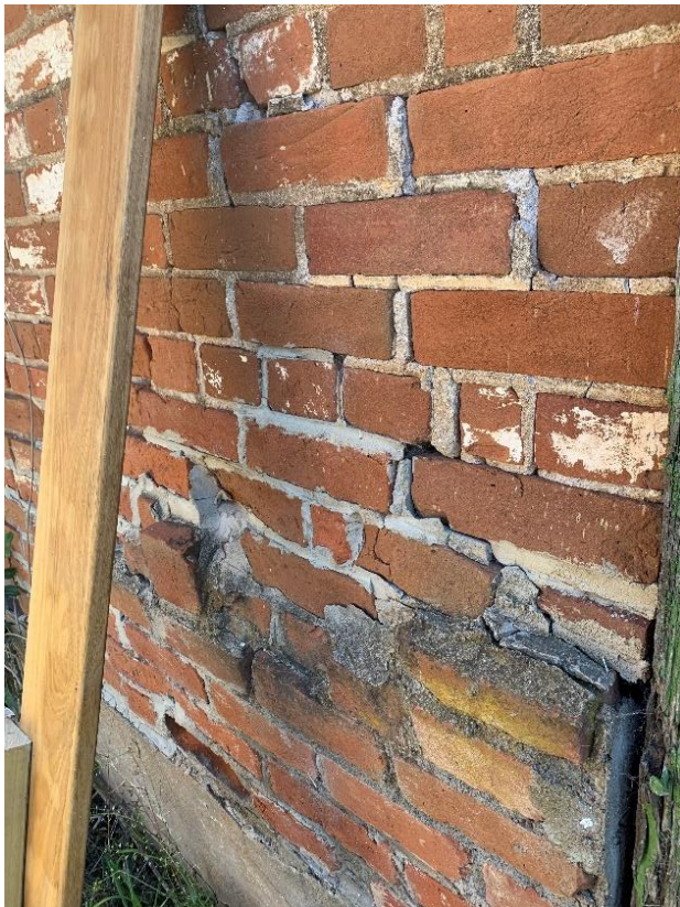
Figure 15. The cracking and bulging of brickwork typical at Negoa, resulting from ground movement. Note the previous cement mortar repairs are failing. Photograph taken September 2020.
