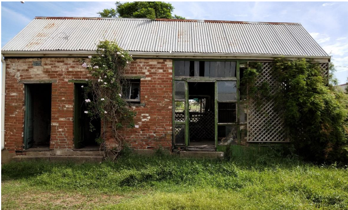
Figure 19. The servants’ quarters at Negoa in April 2018, showing the separate brick and timber sections.
