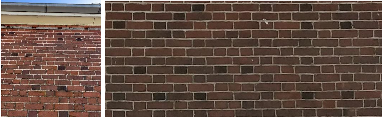
Figure 46. Detail of the brickwork on the southern elevation of the 1840s brick section of the homestead showing the typical Flemish bond (alternating headers and stretchers) and flush pointing
