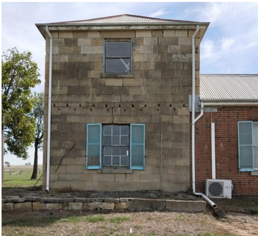
Figure 12. The southern elevation of the c.1850s–60s sandstone section of Negoa, showing the original lower floor window and the non-original upper floor window. It is noted that there is currently no access from the upstairs rooms to the location of the former verandah on this southern elevation. Photograph taken April 2018.
