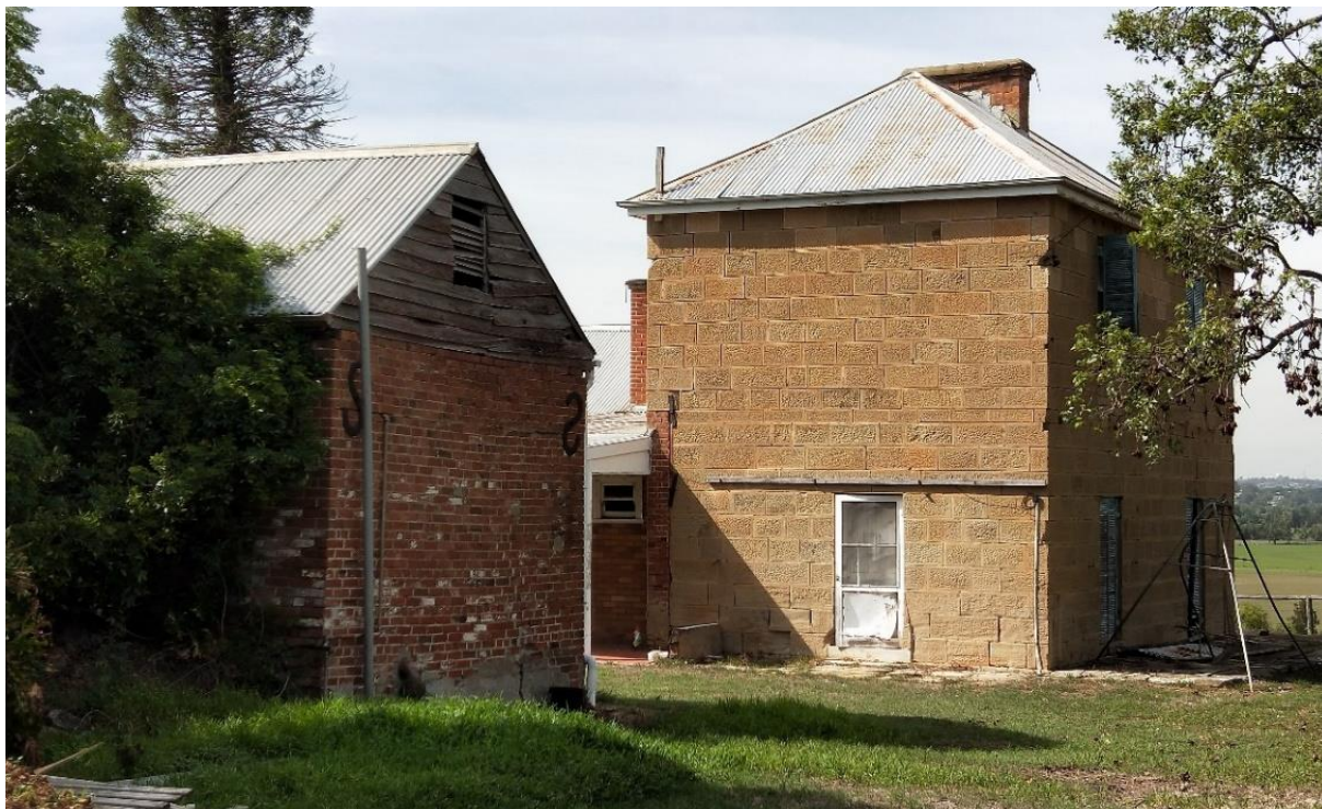
Figure 9. The c.1850s–60s sandstone section of the homestead (right) and the servants' quarters (left). Photograph taken April 2018.
