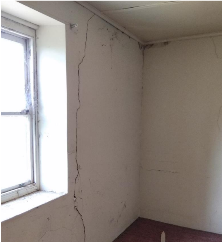
Figure 29. Interior view of one of Negoa's rooms, showing possible structural cracking typical in the internal walls of the c.1850s–60s sandstone section. Photograph taken April 2018.
