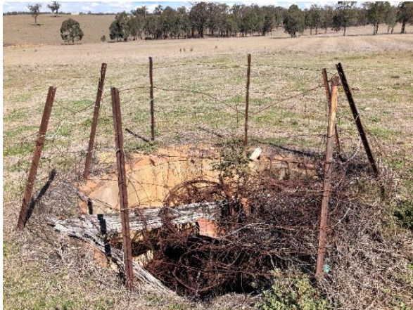
Figure 6. The underground tank at Devine's, constructed of brick and lined with plaster (Source: Extent Heritage 2018).
