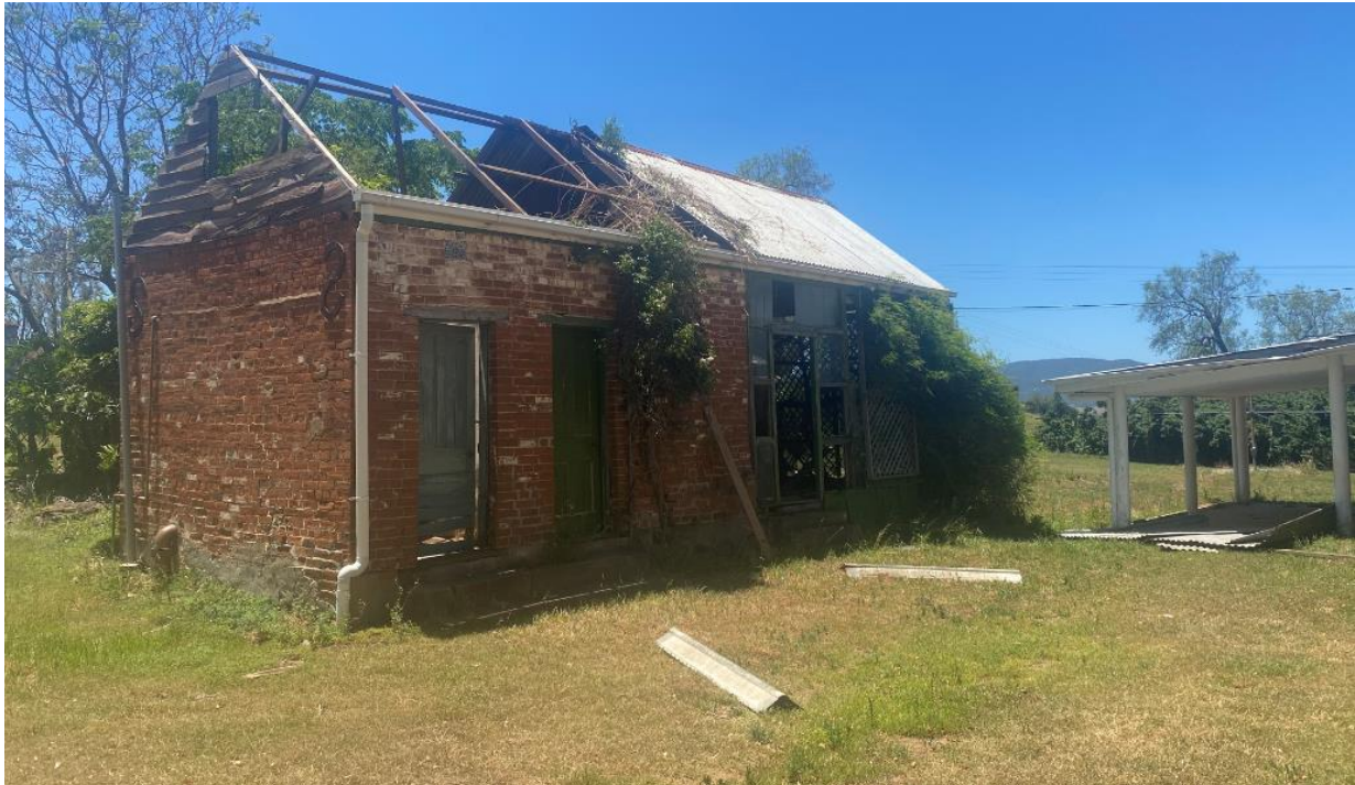
Figure 22. The servants' quarters, showing some of the damage sustained to the roof as a result of a storm event in December 2020.
