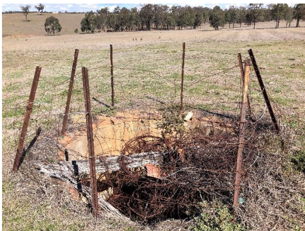
Figure 8. The underground tank at Devine's, constructed of brick and lined with render (Source: Extent Heritage 2018).
