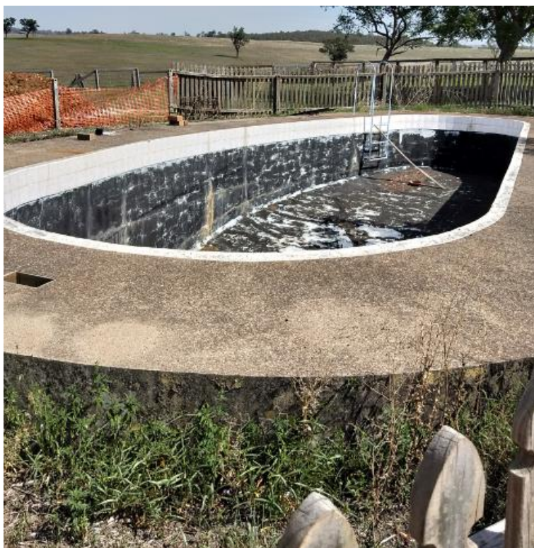
Figure 18. View of the swimming pool and some of its timber paling fencing. This photograph was taken in April 2018; however, the swimming pool has since been backfilled, the fence removed, and the area rehabilitated.
