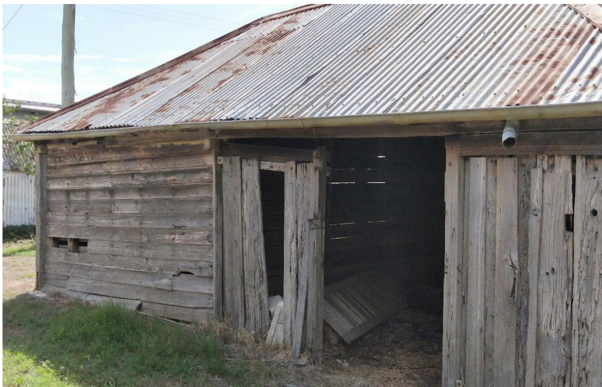
Figure 24. The weatherboard shed at Negoa, constructed from recycled timber materials. Photograph taken April 2018.
