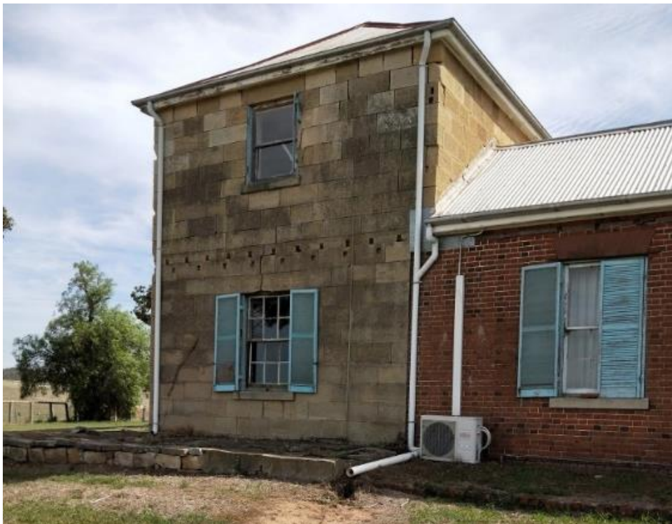
Figure 47. The white downpipes and air conditioning materials detract from the aesthetic appearance of the southern elevation. The air conditioners should be removed and the downpipes replaced with galvanised ones.
