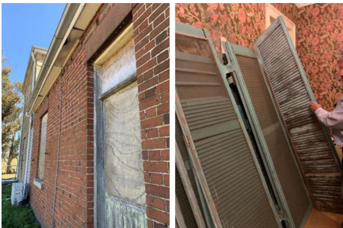
Figure 39. Left: The existing external shutters have been removed, and door and window openings along the southern elevation have been boarded with plywood sheets. Right: The removed external shutters stored inside for repair window.
