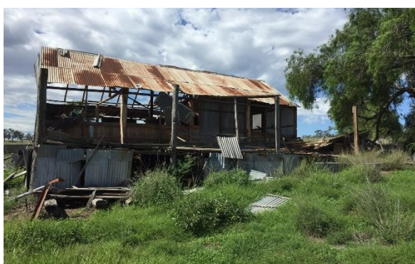
Figure 10. Another view of the damaged remains of the shearing shed at MP27, early 2019 (Source: MACH 2019 in Extent Heritage 2020, p. 94).
