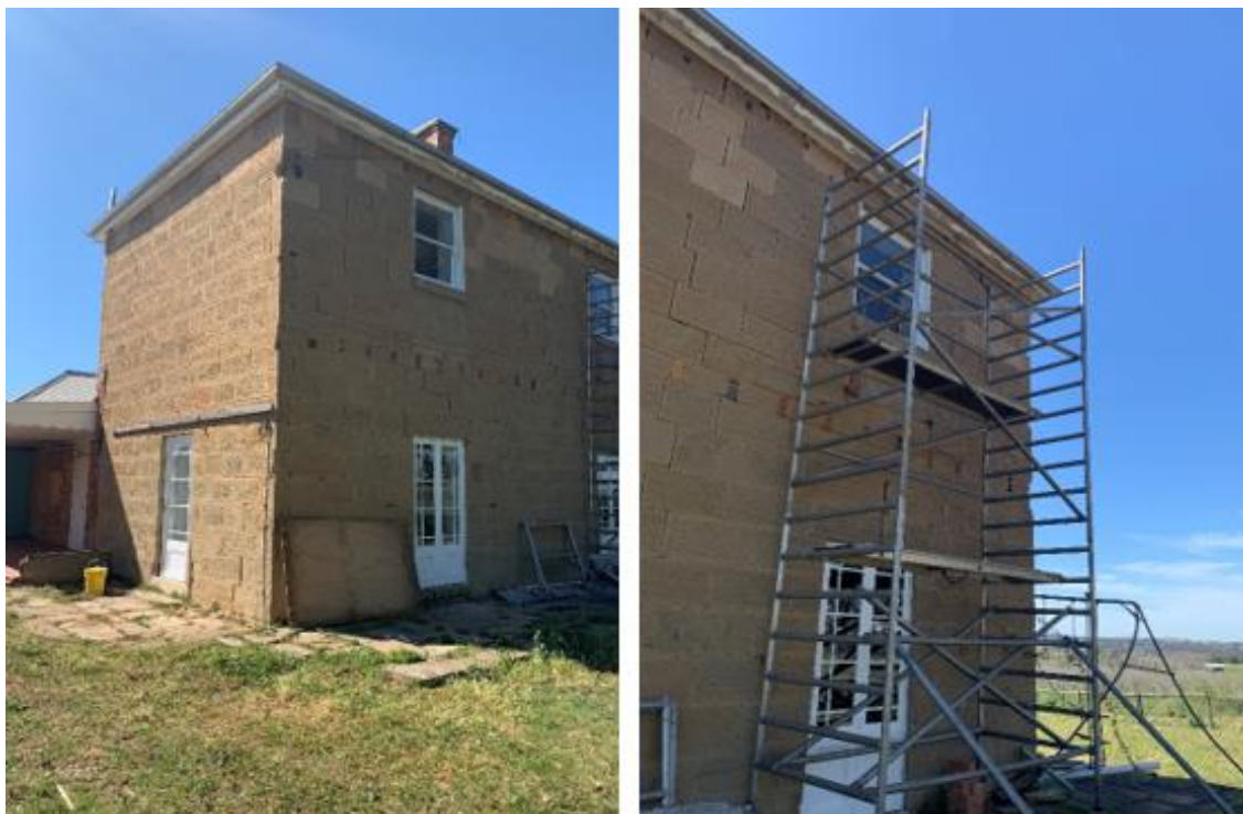
Figure 38. External view of the sandstone section showing the replaced timber doors and windows on the northern and western elevations.
