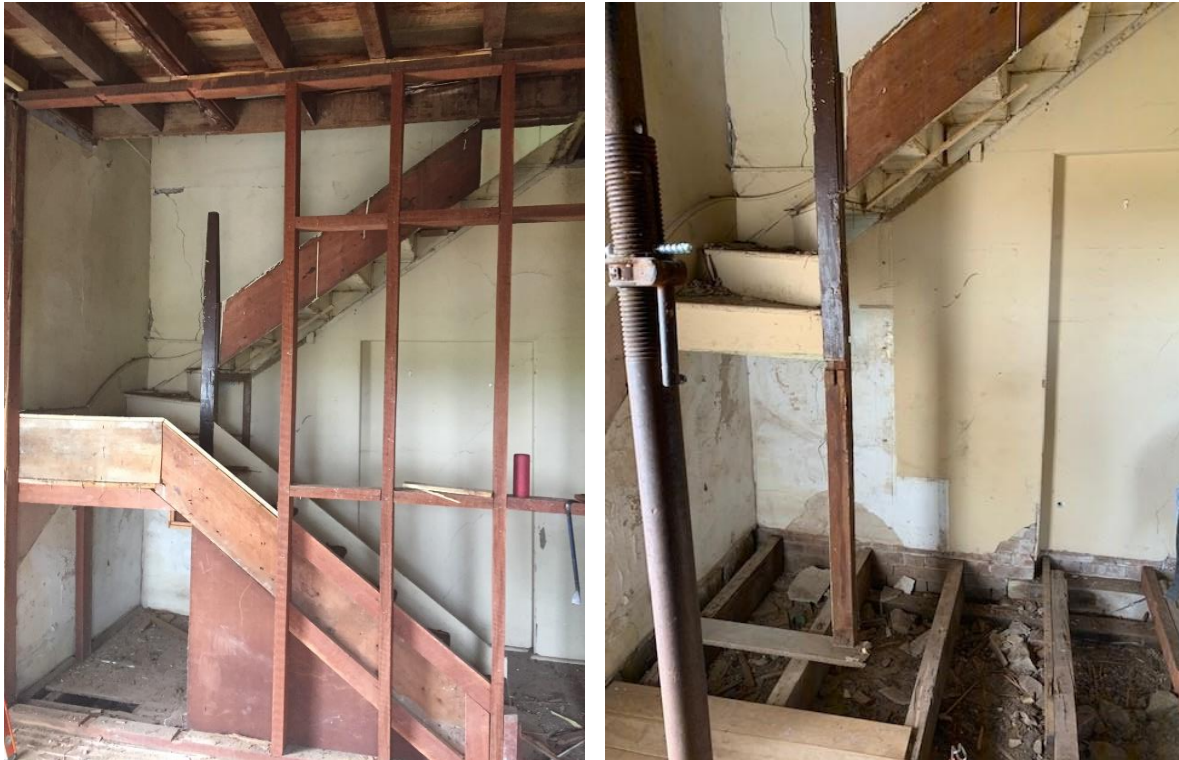
Figure 34. Detail of the termite-damaged timber stairs, since removed and reconstructed.
