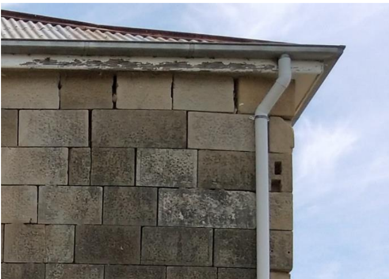
Figure 51. Southern elevation of the sandstone section of Negoa, showing damage to the upper courses of stonework caused by building movement. The causes are to be investigated and the stones reset.
