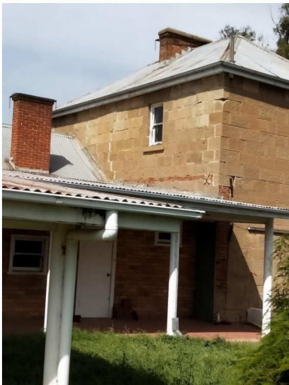
Figure 14. The eastern elevation of the c.1850s–60s sandstone section of Negoa. Photograph taken 2018.
