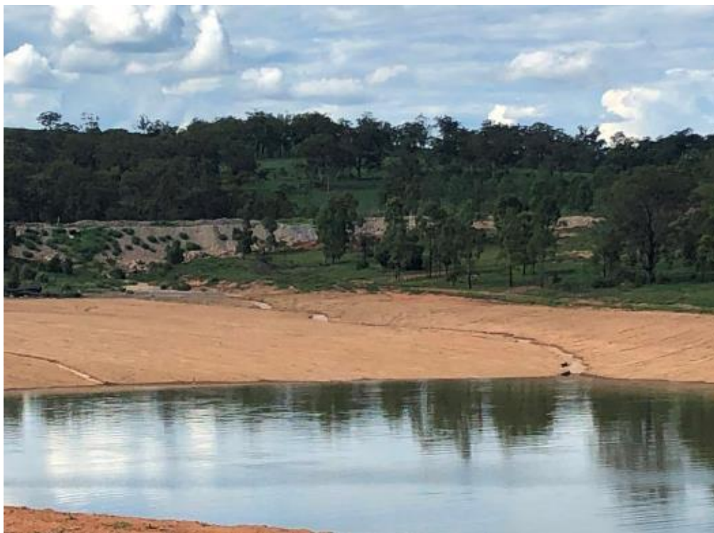
Erosion Photo 16 - Erosion in the Mine Water Dam. Since the site inspection the area has been remediated
