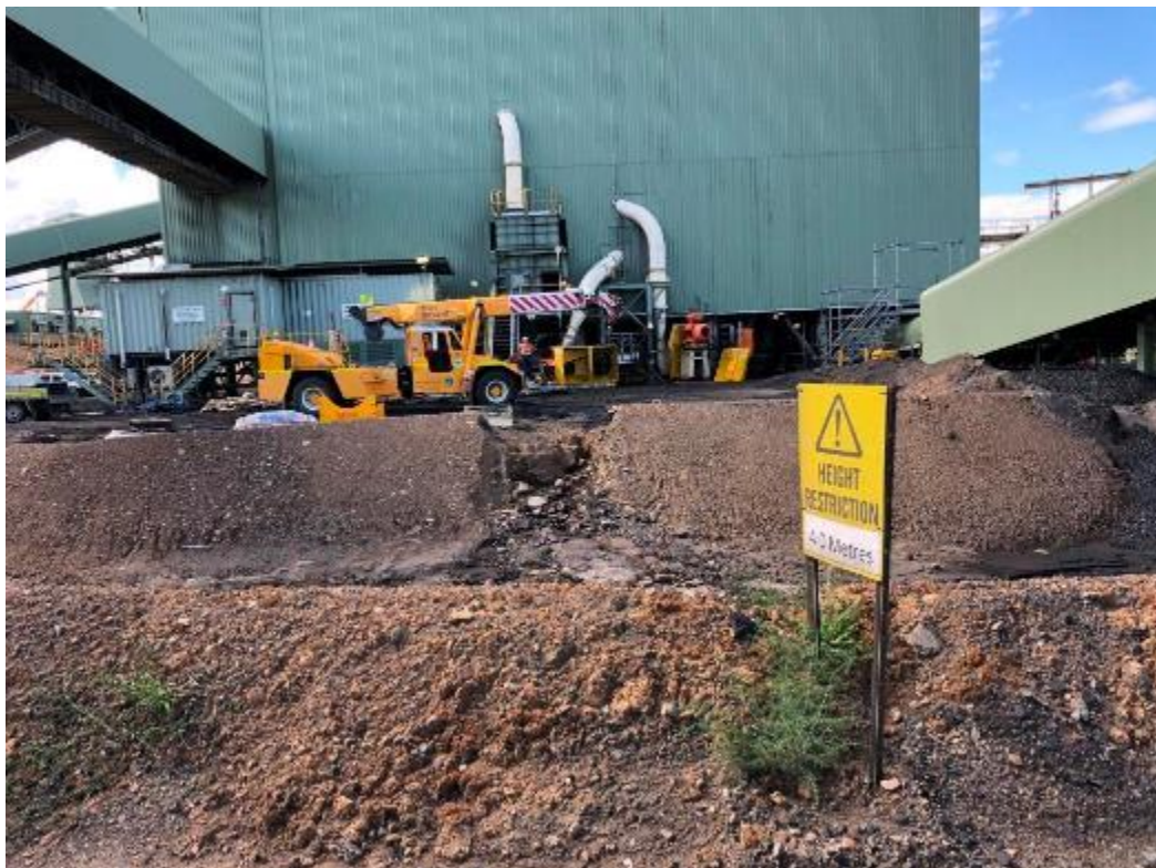
Erosion Photo 6 - Erosion at CHPP
