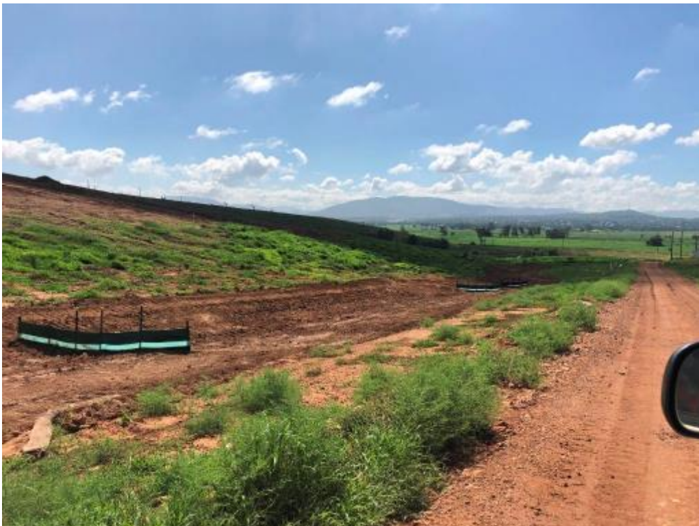
Erosion Photo 2 - Sediment fences within the drain may fail as sediment fences have been used in an area of concentrated flow
