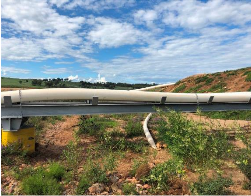
Water Management Photo 17- Fines disposal pipeline cross the cleanwater drain. Note, evidence provided since audit inspection of the installation end of line burst protection flow meters.
