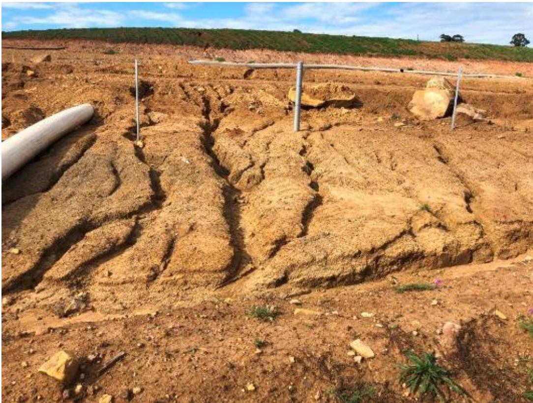
Erosion Photo 10 - Erosion within the fines emplacement area. Within the dirty water catchment.
