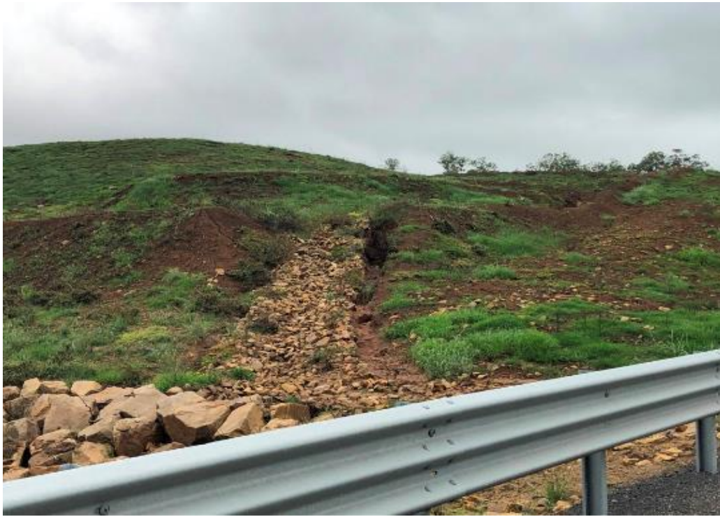
Erosion Photo 15 - Blow out and erosion of rock drain on left hand side of the entrance road
