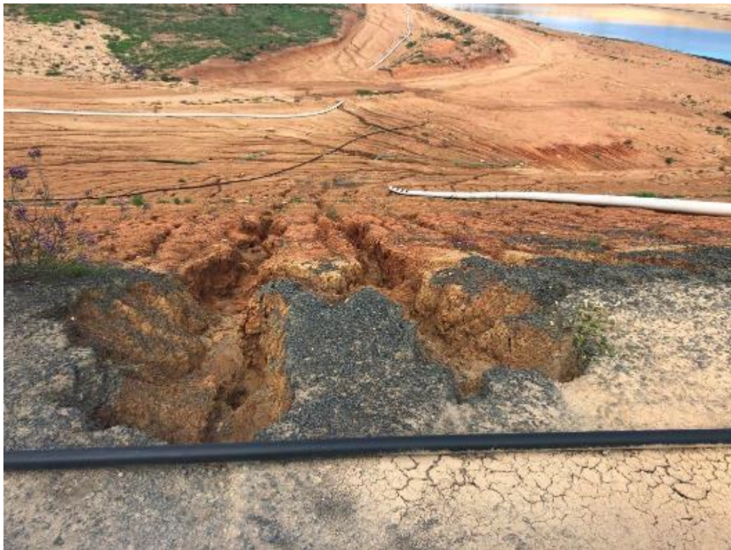
Erosion Photo 12 - Erosion of the inside of the wall of the fines emplacement area
