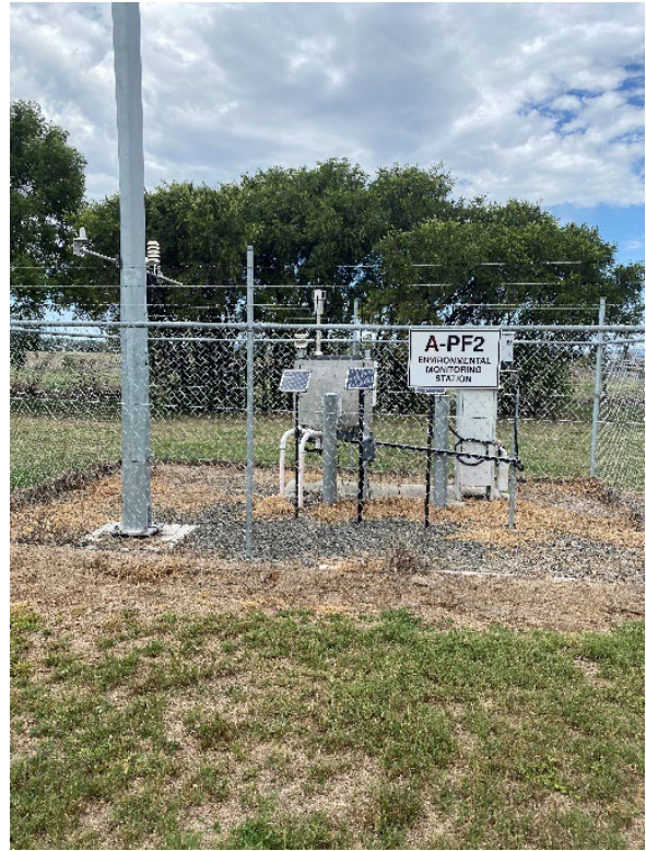
Photograph F.35 Meteorology station
