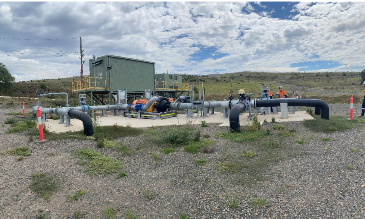
Photograph F.36 Water pump infrastructure
