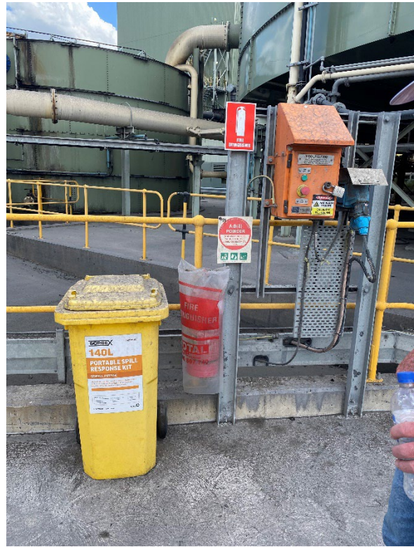
Photograph F.55 Spill kit and fire extinguisher
