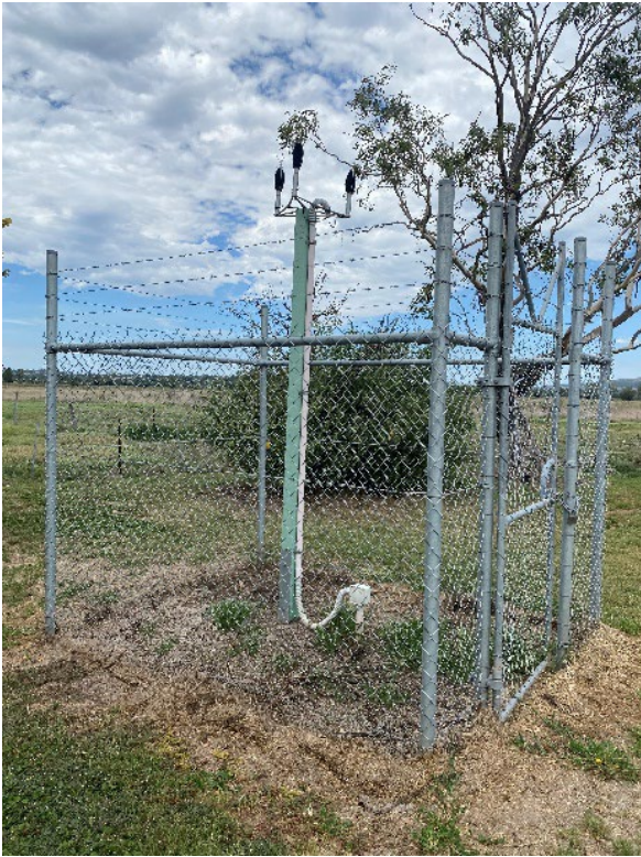
Photograph F.34 Meteorology station
