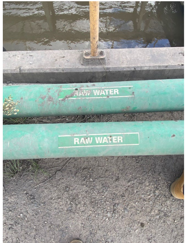
Photograph F.105 Water management system
