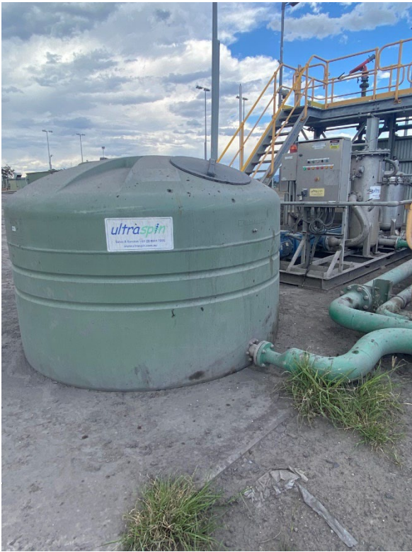
Photograph F.102 Oily water separator
