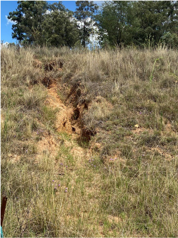
Photograph F.51 Erosion
