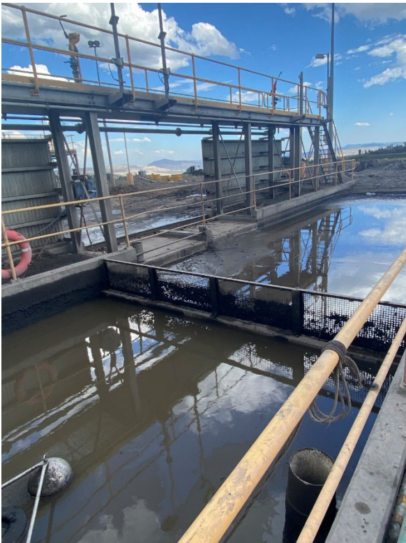
Photograph F.104 Oily water separator
