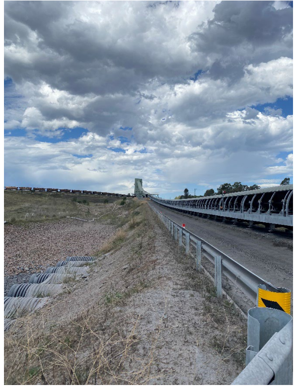
Photograph F.71 Coal conveyor
