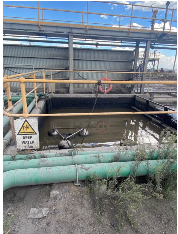
Photograph F.103 Oily water separator
