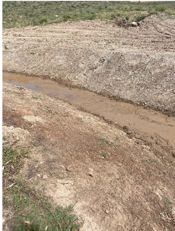
Photograph F.29 Surface water drainage to SD3
